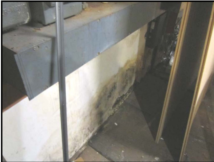
INTERIOR VIEW OF WATER DAMAGE WITH POSSIBLE MOLD ON SOUTH WALL NEAR LOADING DOCK
