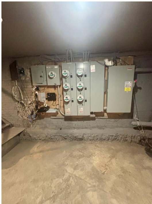
Individual Electric Meters & Panels
