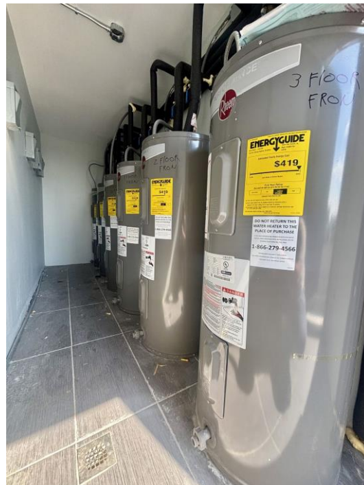
Individual Water Heaters (Roof Closet)
