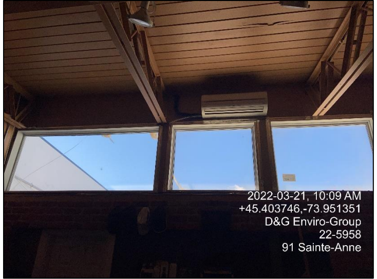
Photo 6 – Air conditioning unit located in one of the commercial units.
