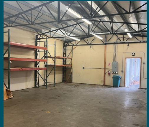
Warehouse with 3 Phase power
