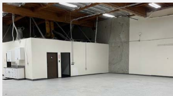
Warehouse lighting & Distributed power
