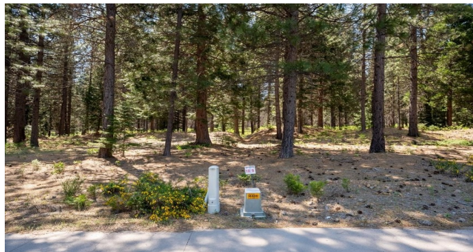
Utility pedestals stubbed at the lot line
