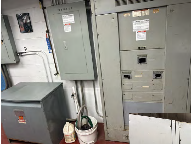
Bldg. A 1,200 Amps at 480 Volts 3-Phase
