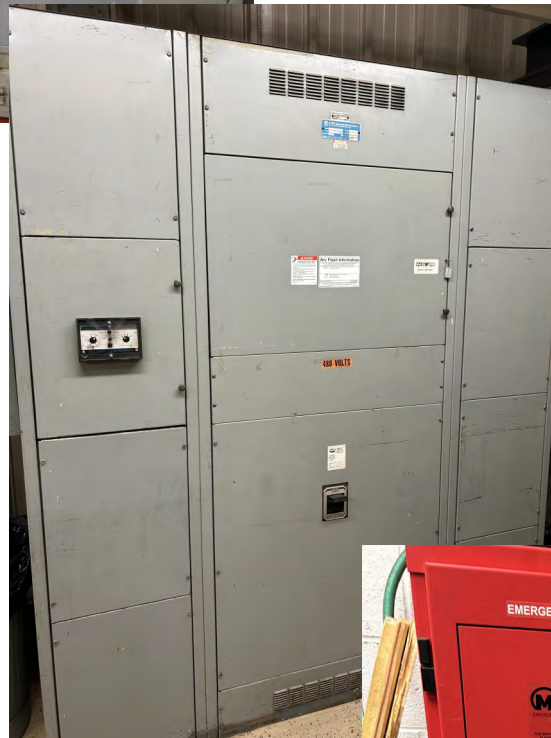
Bldg. B 1,600 Amps at 480 Volts 3-Phase
