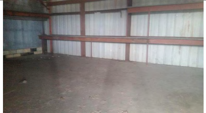
Photograph 28 - View of the former maintenance building on the northern portion of the subject site
