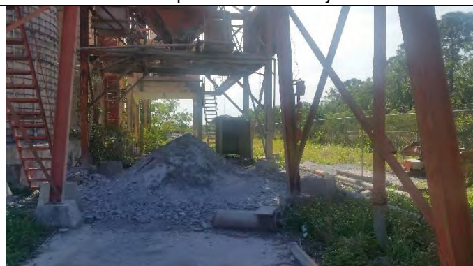
Photograph 15 - View of concrete equipment located on the northwest portion of the subject site
