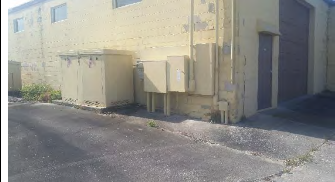
Photograph 19 – View of the pad mounted transformer located on the northeast portion of the subject site
