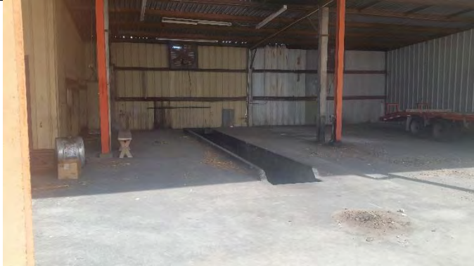
Photograph 27 – View of the former maintenance building on the northern portion of the subject site
