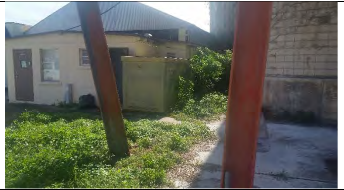
Photograph 18 – View of the pad mounted transformer located on the northwest portion of the subject site
