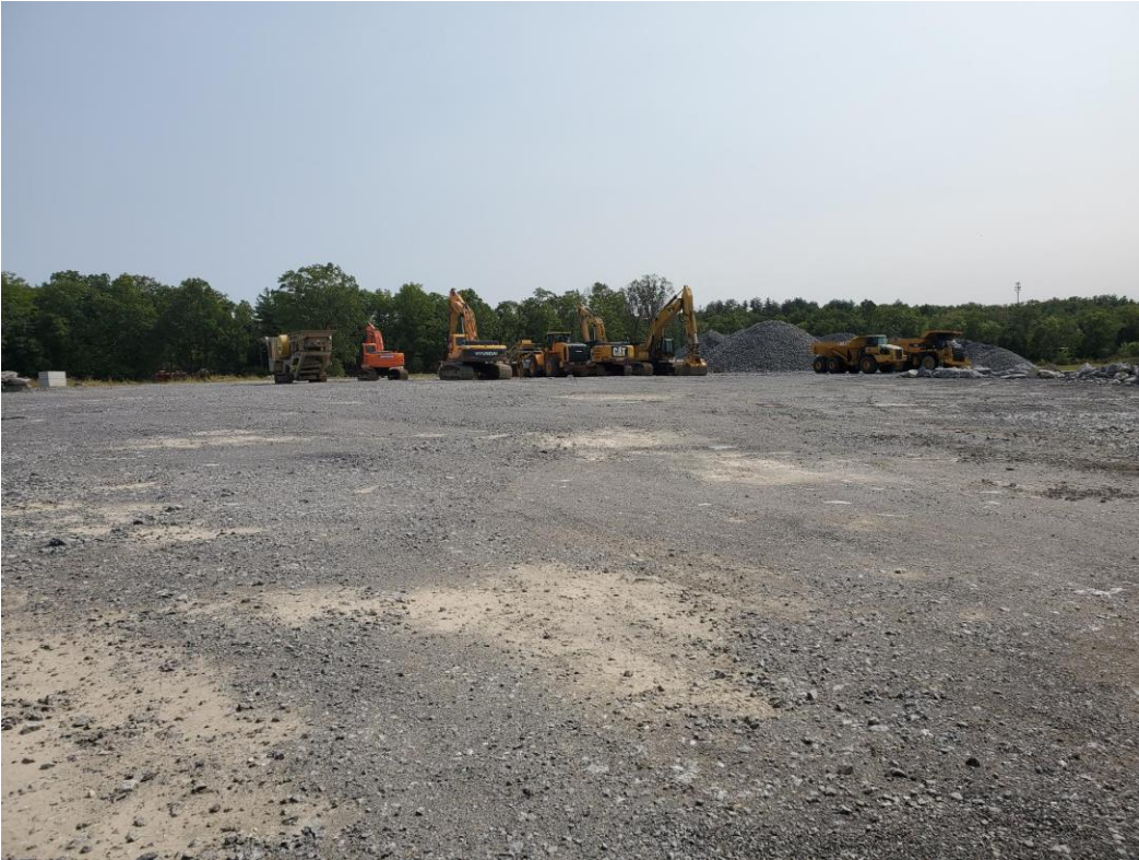
Site with equipment
