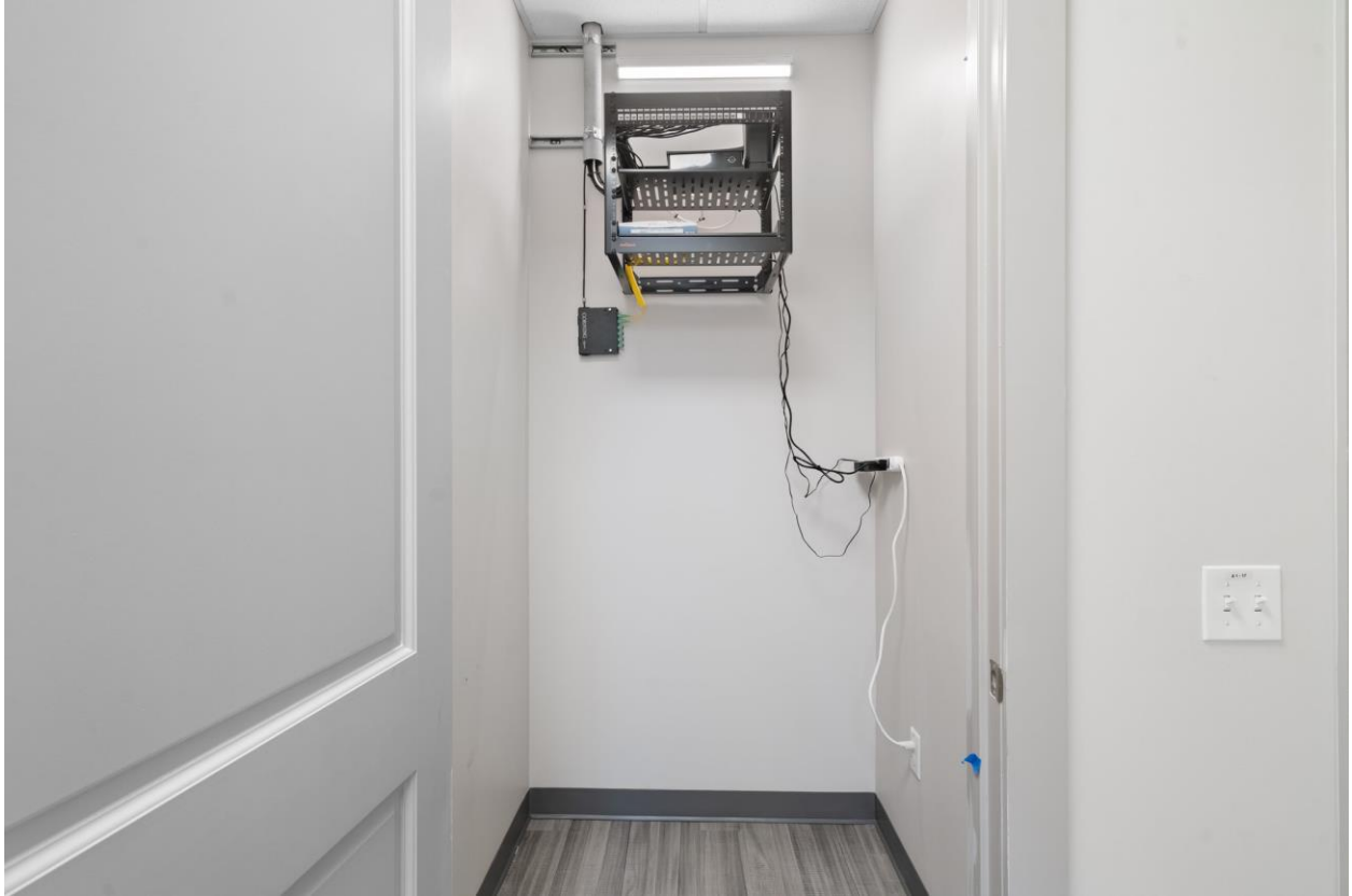
IT Infrastructure room
