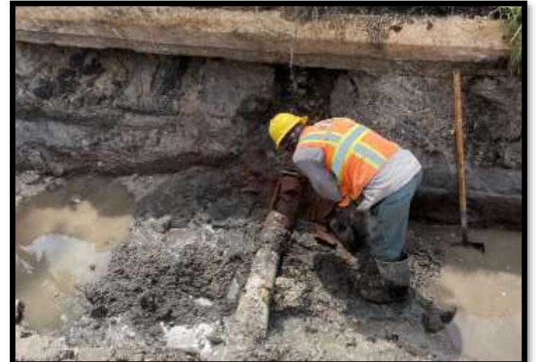
Sewer lateral conflicts
