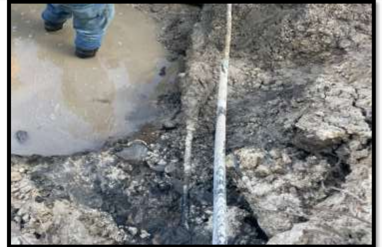
Gas line conflict
