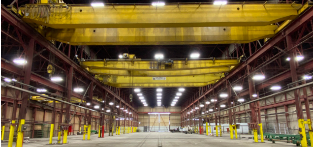
EAST-WEST CRANE BAY: (2) 30 TON CRANES; (2) 25 TON CRANES
