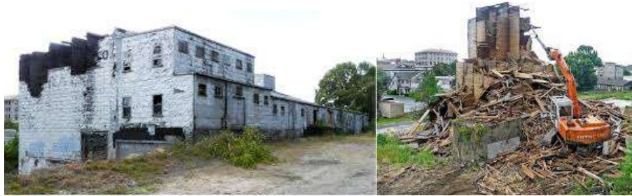
Figure 3: The dilapidated Campbell Grain Building has been demolished leaving a site ready for development
