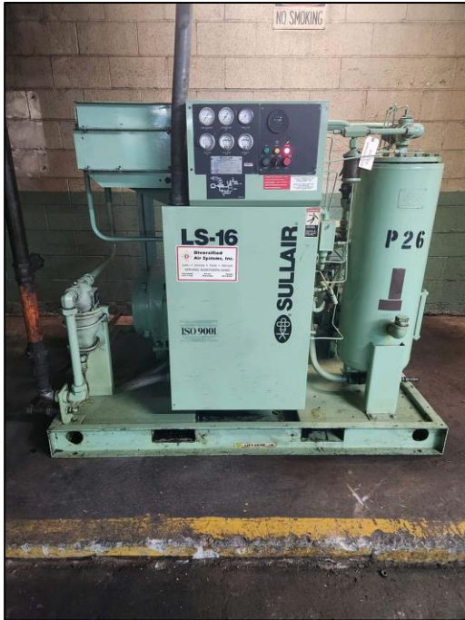
Air compressor – rebuilt in 2023
