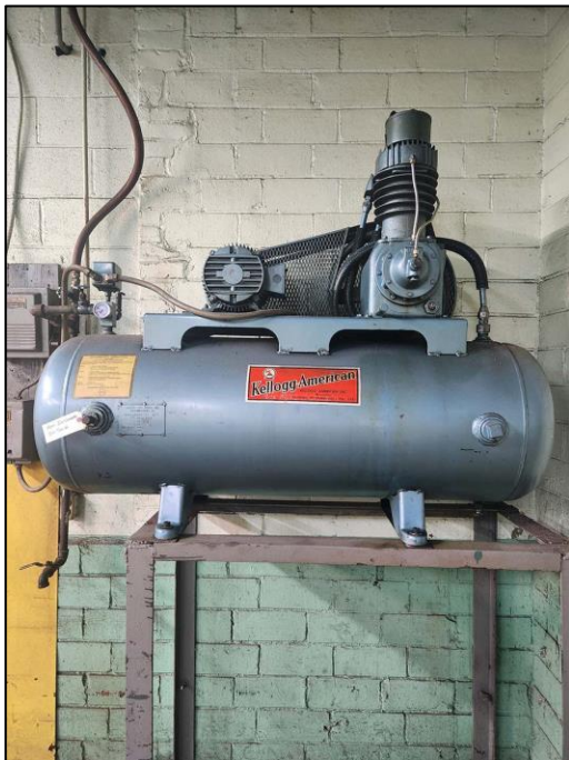
Auxiliary Air compressor
