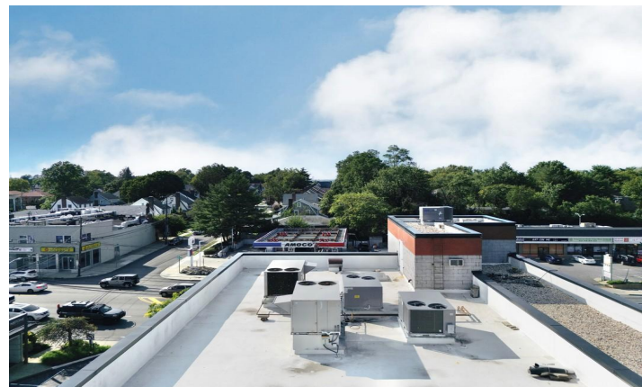
Redundant Rooftop HVAC & New Roof
