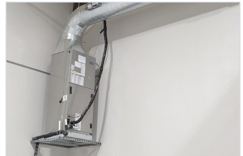
Dedicated Warehouse A/C
