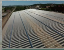
160KW SOLAR ROOFTOP
