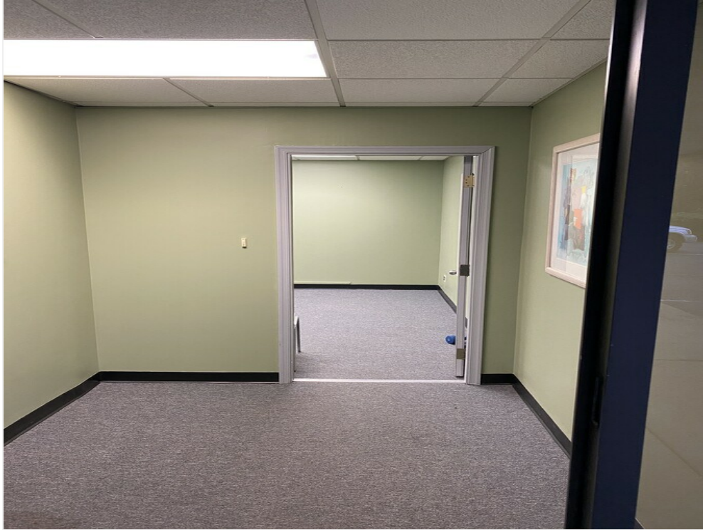
Looking from front door or suite, past foyer to entrance to suite
