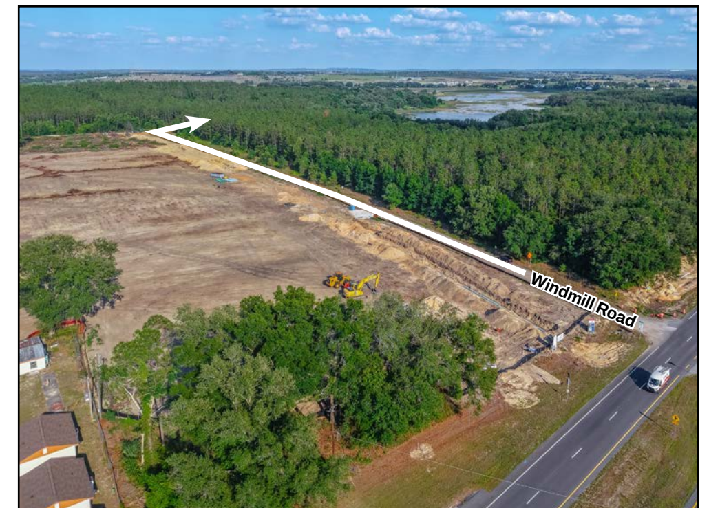
From US 27 and Windmill Road leading to the property's southern entrance. Highland Pines community is cleared for construction.
