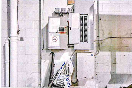
Utilities with electric panel
