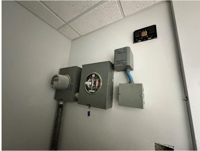
Electrical Closet – First Floor
