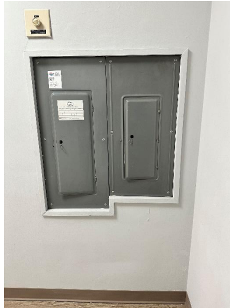
Suite B – Electrical Panel
