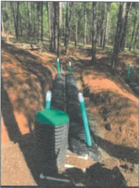
Figure 1: Upper STA Area with Inspection and Valve Access Risers
