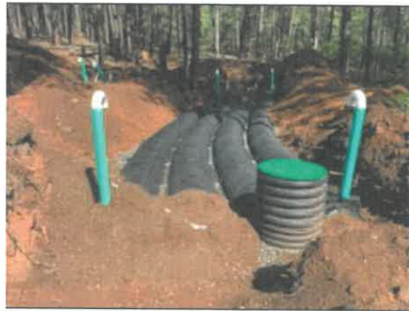
Figure 2: Lower STA Area with Distribution Valve Risers, Inspection Risers
