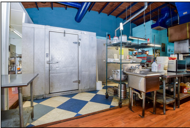
Main Level Walk-In Freezer & Refrigerator
