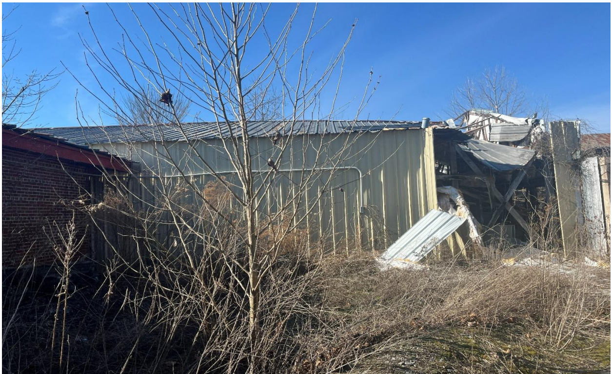
Exterior (Damage to Rear of Building)
