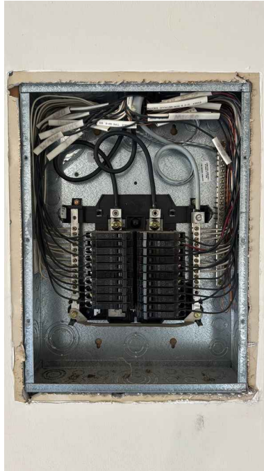
Sub Panel Garage
