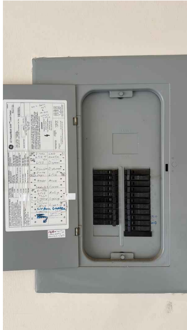
Sub Panel Garage
