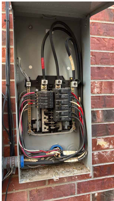
Main Panel Right Side Of Home
