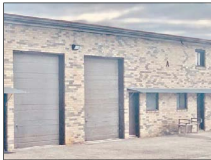
Dock High Doors C7 & C8
