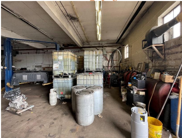
Recycled oil used for heating
