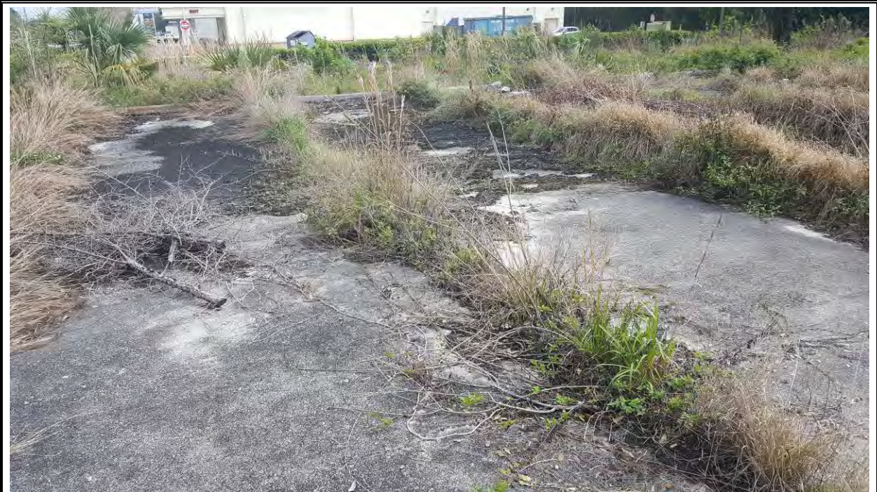
Photograph 3: View of a concrete paved areas located on Parcel 1 of the subject property.
