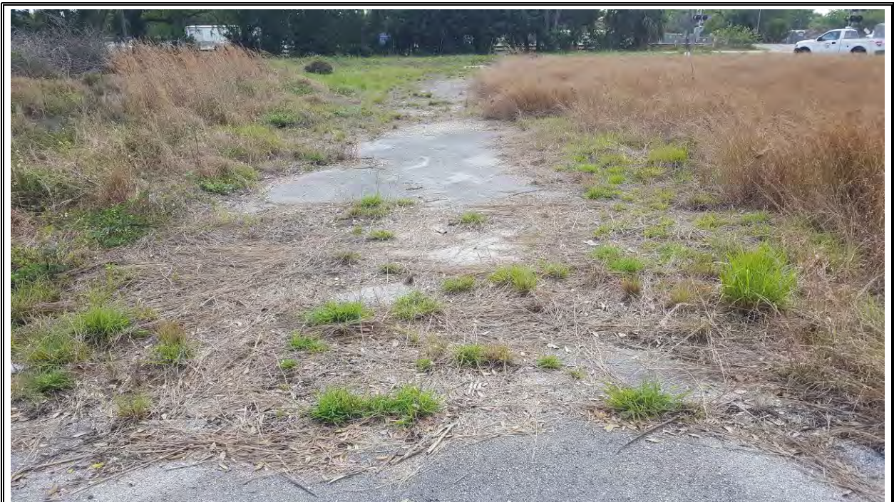
Photograph 2: View of a concrete paved area located on Parcel 1 of the subject property, looking south from US Highway 92.
