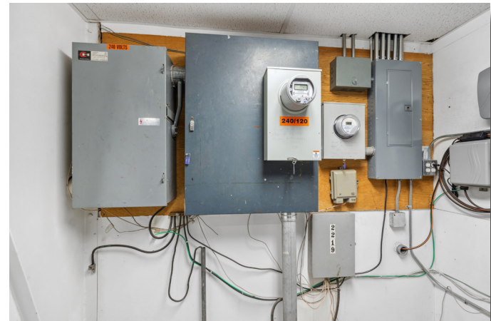
Electrical Panel B
