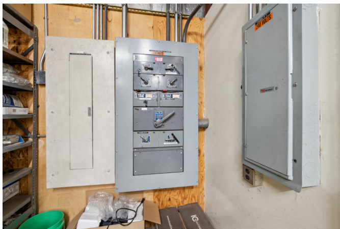
Electrical Panel A
