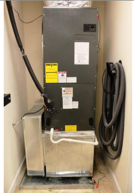
Individual HVAC Units so tenant controls thermostat
