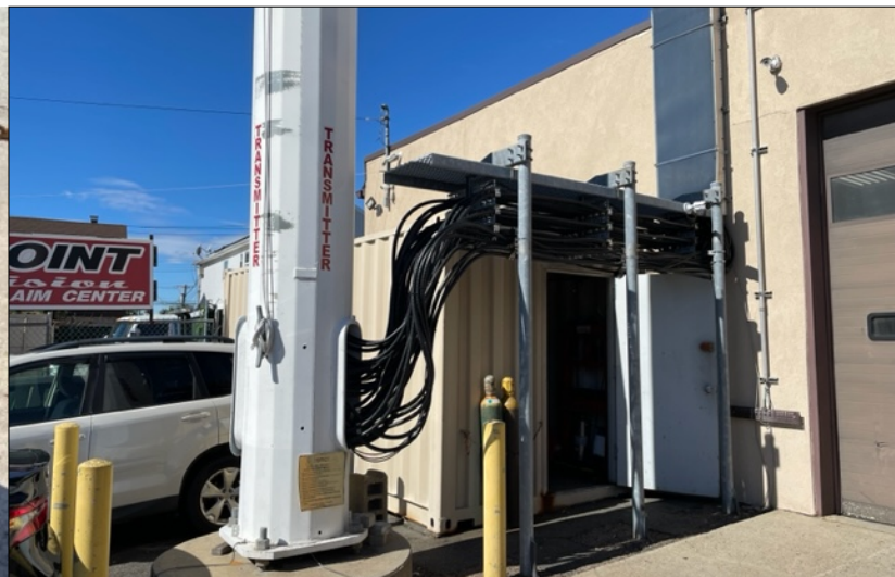
T Mobile Cell Tower
