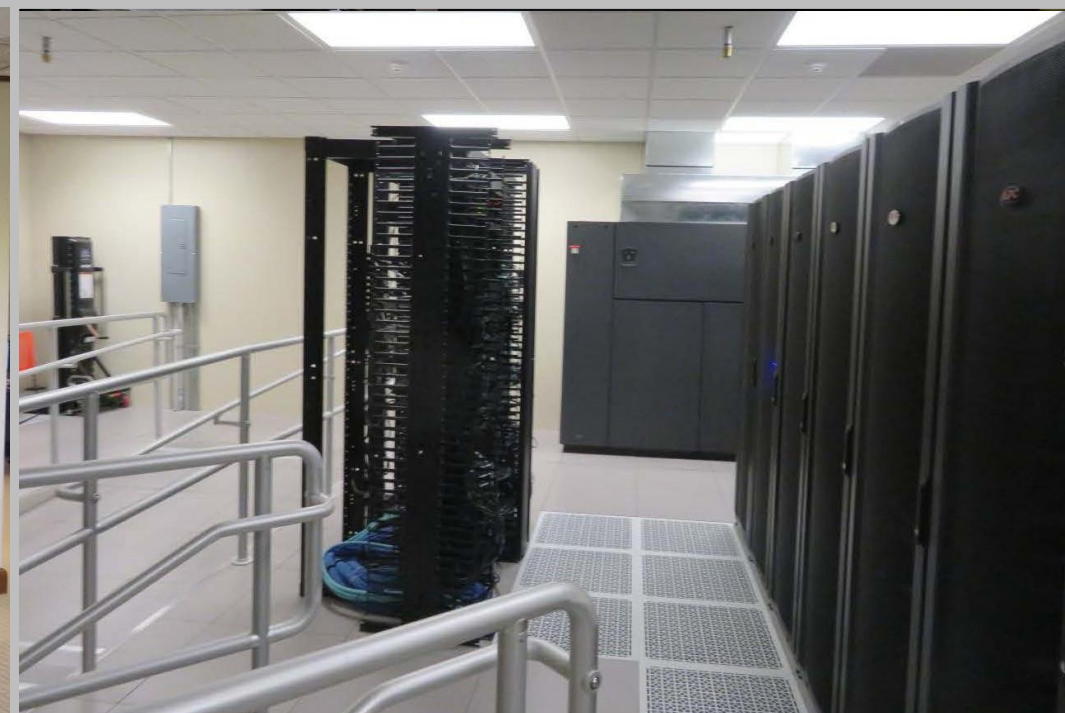
DEDICATED IT SERVER ROOM
