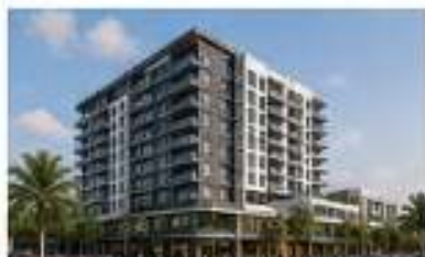
21 HOLLYWOOD 2100 N Federal Highway 14-STORY MIXED-USE 200 RESIDENTIAL UNITS UNDER CONSTRUCTION (EST. COMPLETION 2026/27)
