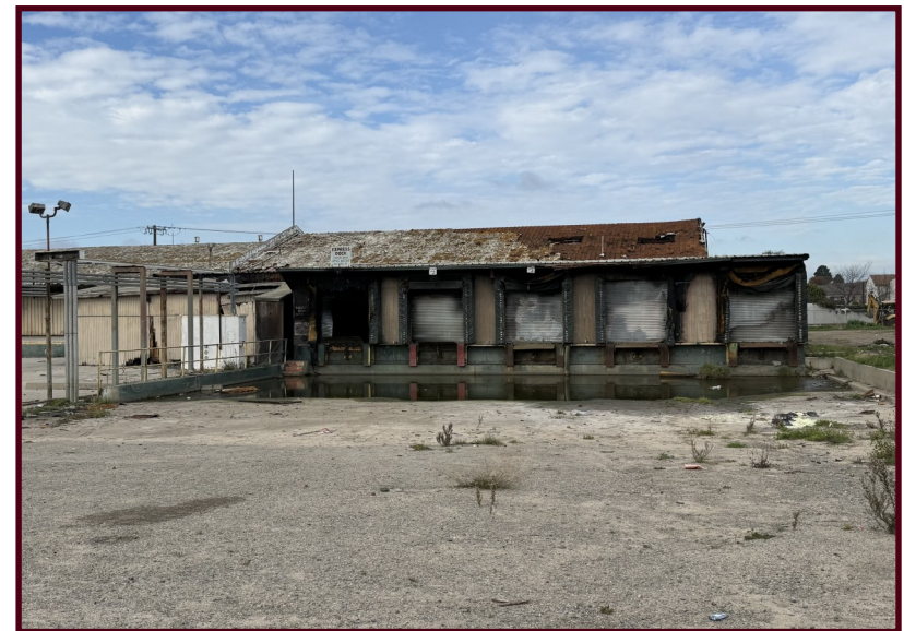
South Side of Fire Damaged Portion of Warehouse
