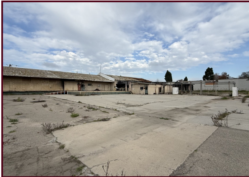
Fire Damaged Portion of Warehouse is on the far end
