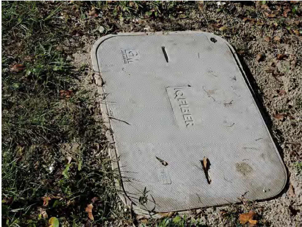
Fiber Optics (1) at Frontage
