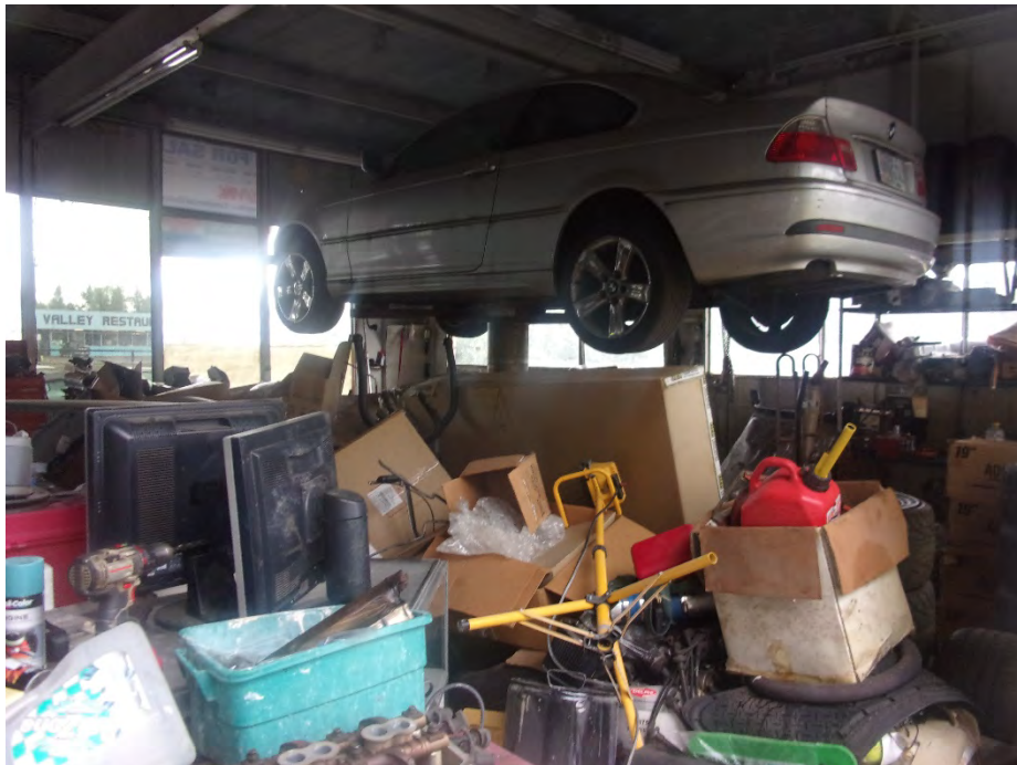
Photo 6. One of two inground hydraulic lifts located within the automobile shop.
