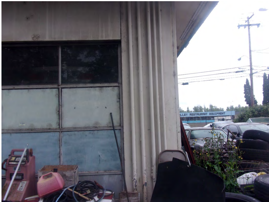
Photo 8. Old vent pipes that were once connected to the five underground storage tanks located to the north of the auto shop.
