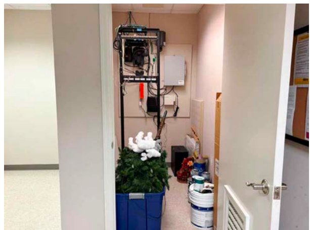
North Space - Utility Room
