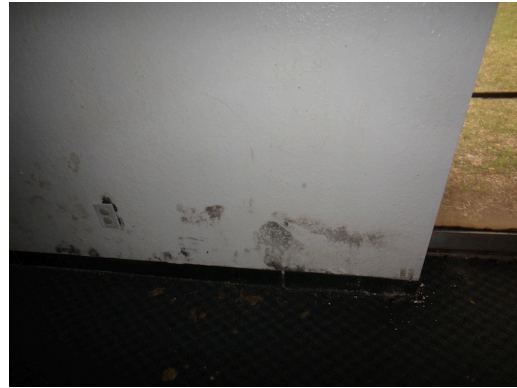
Moisture damage bldg 2
