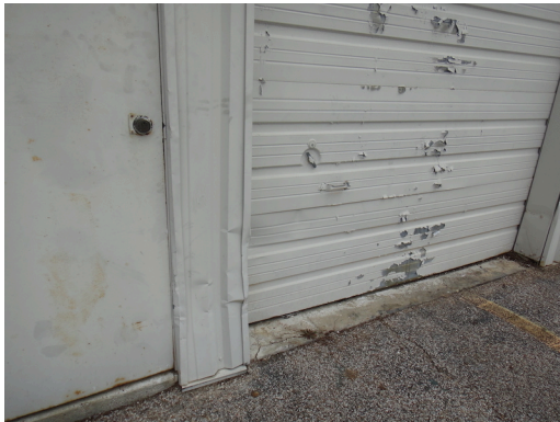
Fair to poor finishes
