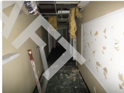
Bldg 2 interior poor
