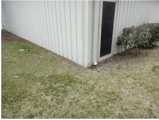
Poor drainage along southeast
