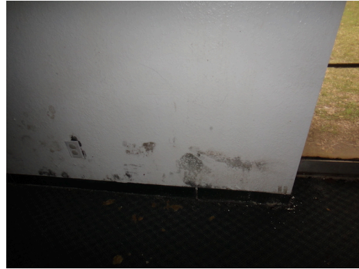
Moisture damage bldg 2
