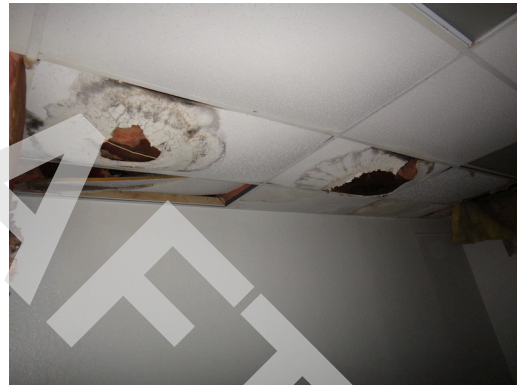
Past roof leaks bldg2
