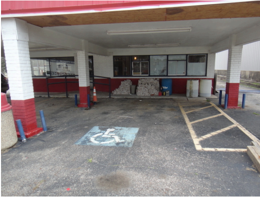
ADA signage needed
