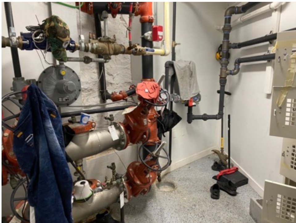
Sprinkler and Locker Room
