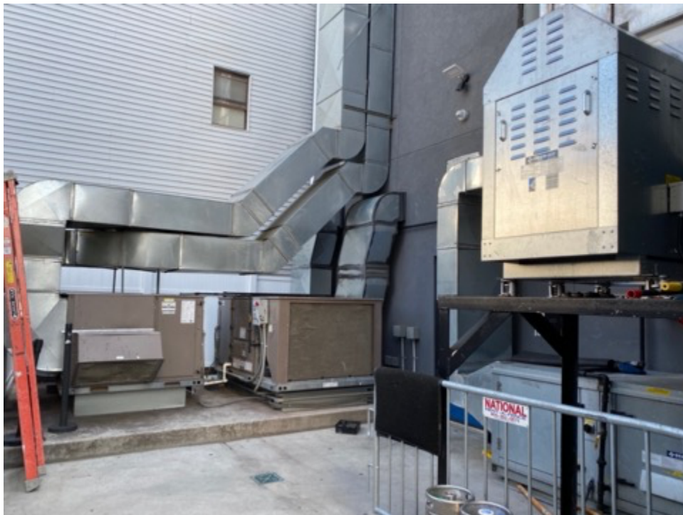
Ventilation and HVAC systems at rear of site
