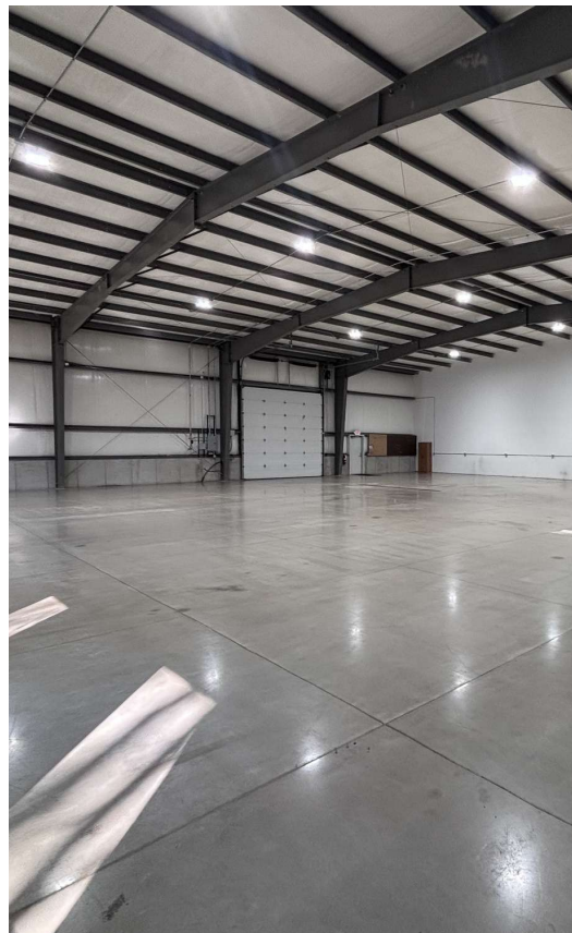
Plumbed for future restroom
