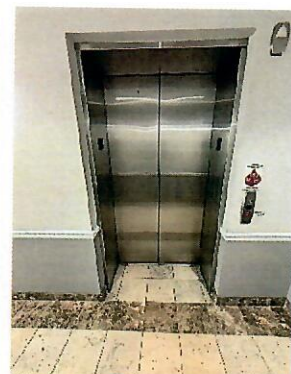
OTIS 3,000 lb. capacity elevator
