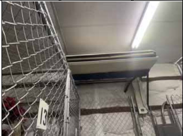
Typical HVAC Blower – 1350 Lake Washington Rd.
