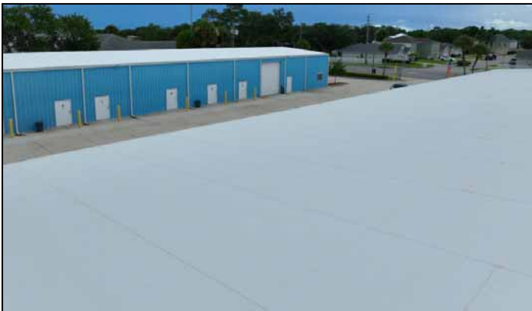
New Roof on Subject Buildings As Viewed from 1360 Lake Washington Rd. Facing Southeast towards 1350 Lake Washington Rd.
