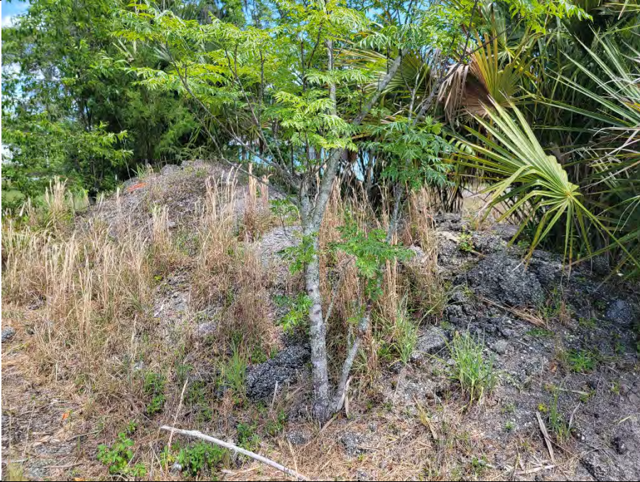
Photograph 13. Asphalt and soil on the western portion of the subject property from the 1996 UST removal.
