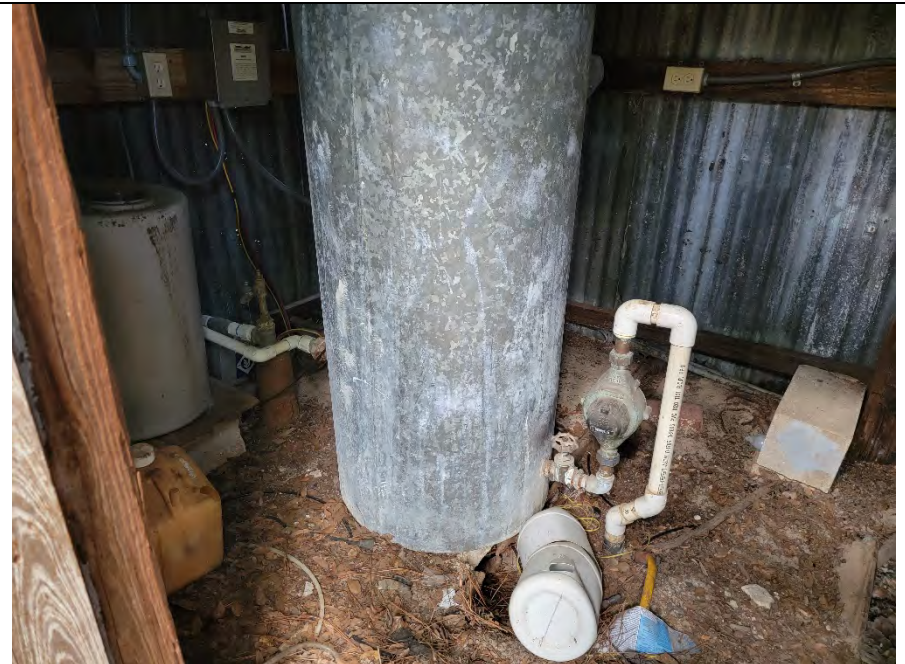
Photograph 16: Water well, chlorination system, aeration tank, and pump system.
