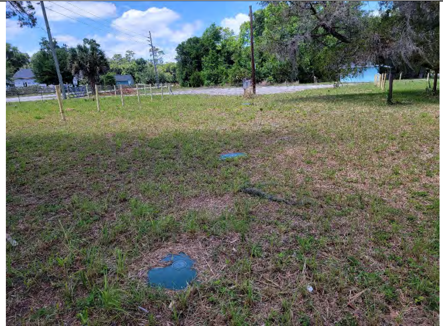
Photograph 10: Septic tank, grease interceptors, dosing tank and pump electrical connection west of the subject property building.
