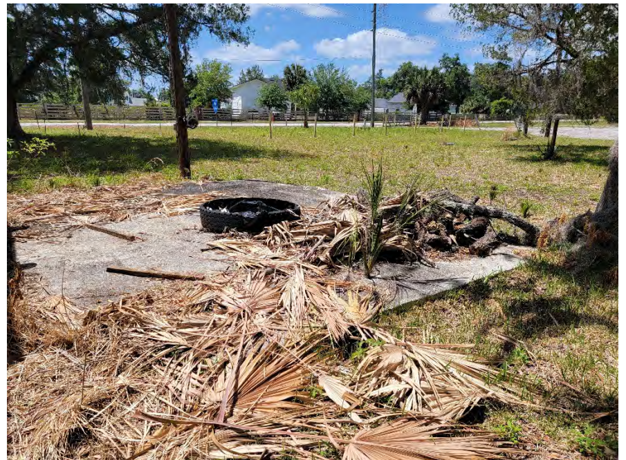
Photograph 8. Concrete building pad on the west side of the subject property building.
