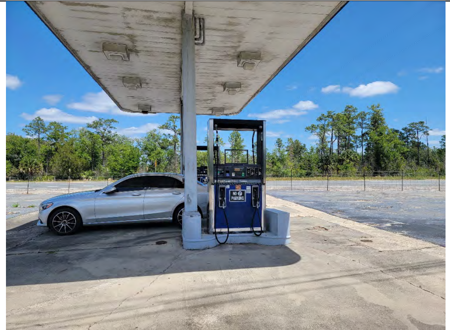
Photograph 2. Fuel dispenser pumps and canopy on the eastern portion of the subject property.
