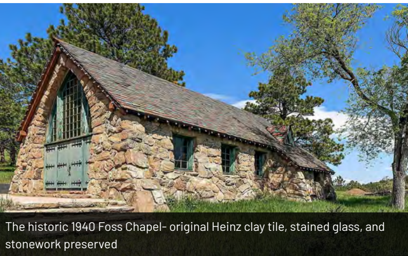
A spiritual and architectural anchor- ideal for reflection, gathering, or heritage preservation
