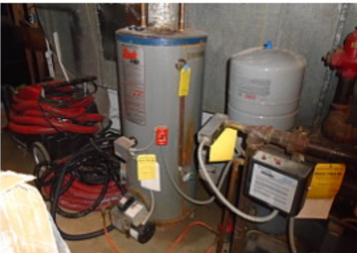
Basement - water heater
