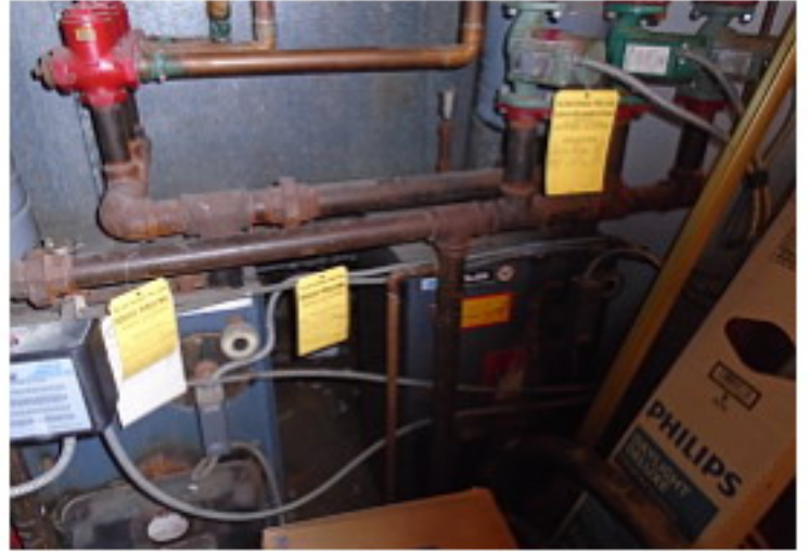
Fuel oil furnace and sprinkler system
