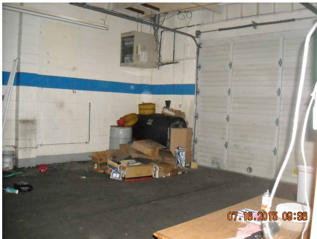
PHOTO 4: Waste oil AST located in the northeast corner of the structure
