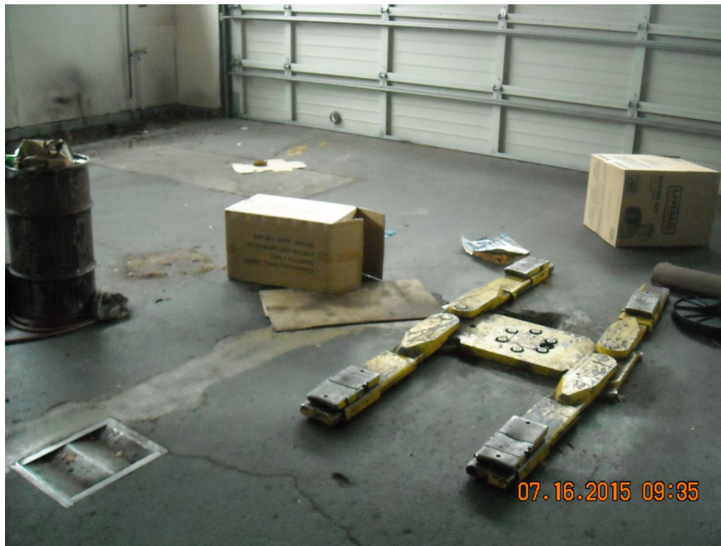
PHOTO 3: In-floor hoists located in the southeast portion of the structure
