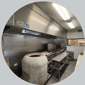
Full Commercial Kitchen
