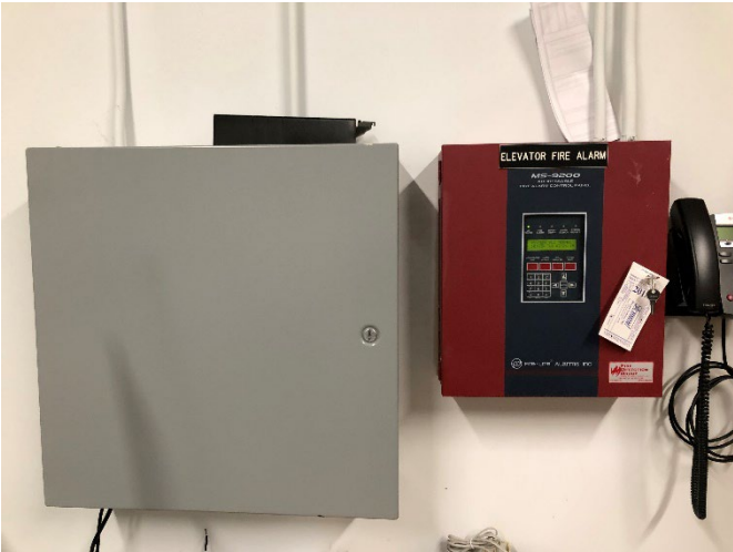
Fire System Panel
