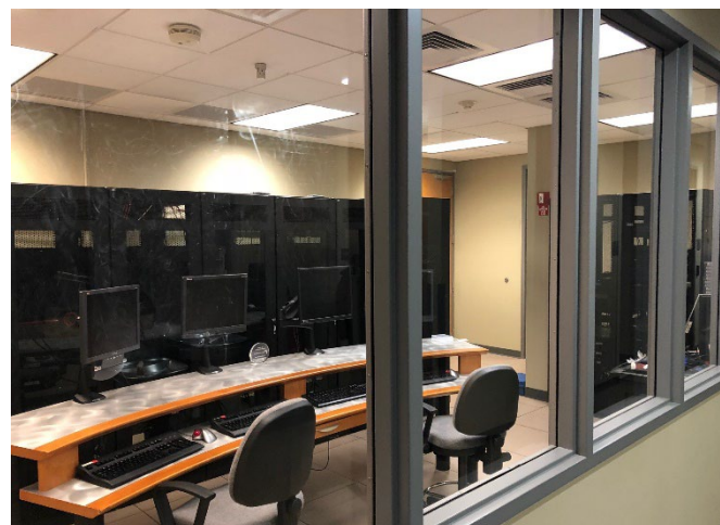
Secured Data Center
