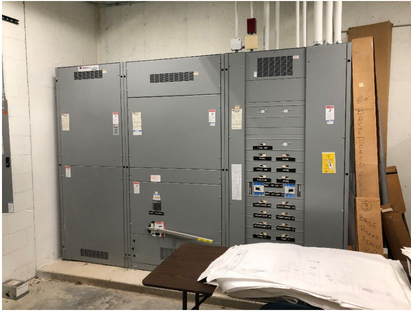
Main Electrical Switch Panels
