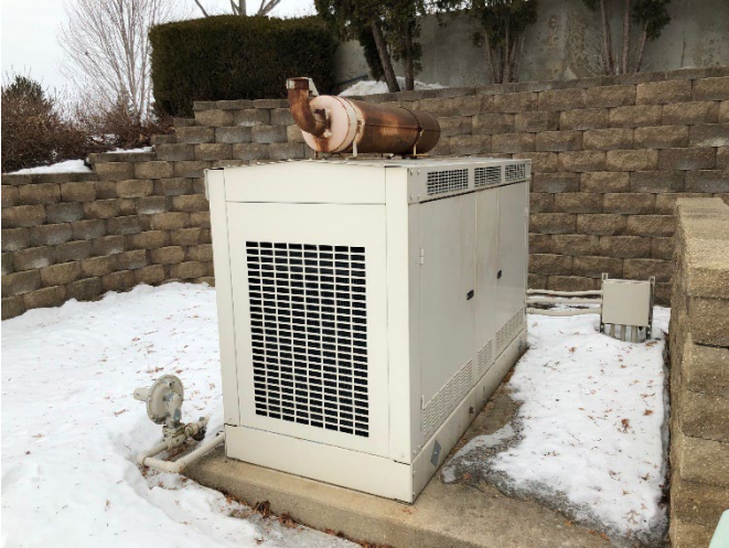
81 Kw Spectrum Brand Generator
