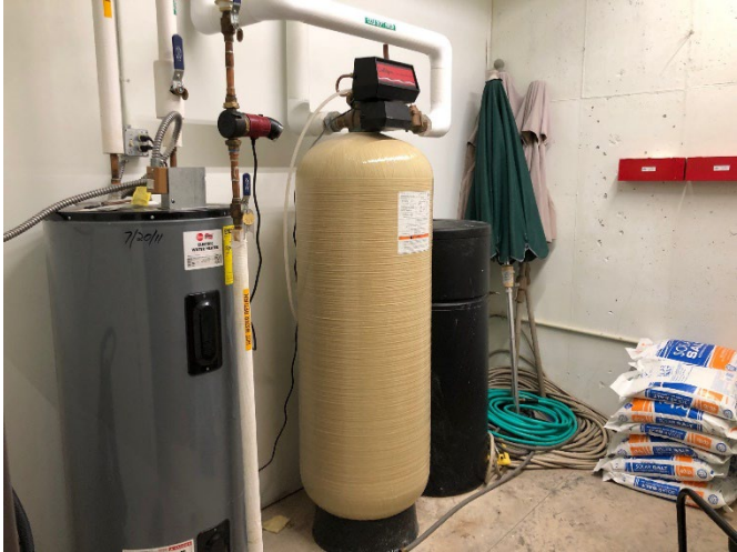
Water Softening System
