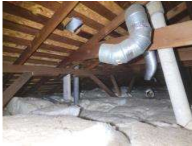
Unhooked vent noted above the main unit near the kitchen.
