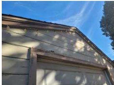
Weathering and decay noted in areas.
