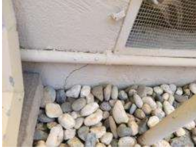
Cracks found at areas of the lower wall/foundation wall.
