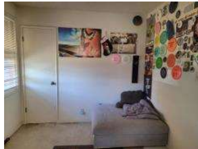
Drywall, cracks General condition appears serviceable. Typical noted, condition
