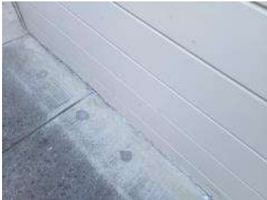
Generally serviceable, Weathering and decay noted in areas
