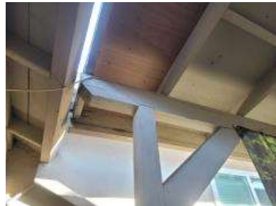
Wood decay and deterioration noted at various areas of the exterior patio.
