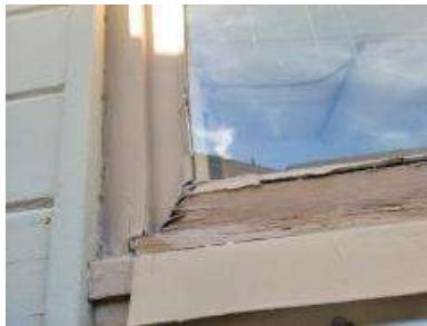
The windows show wood decay and damage in various areas.
