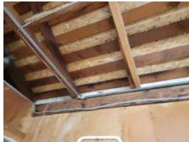
Water stains in various areas.
