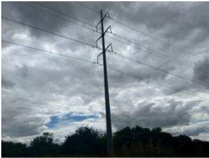
Photo #21 Mideast Overhead Powerlines
